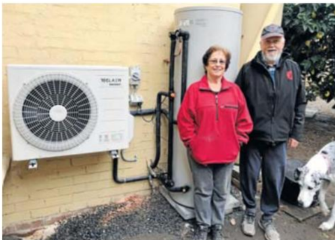
Spencer Field and Annette Trood from Healesville were the first two people to install a heat pump in July 2019 and they are very pleased with the outcome. Picture: SUPPLIED
